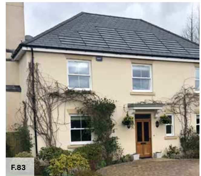
Figure 83: Use of shingle-like solar panels on a slate roof, with the design and colour of the solar panels matching those of the adjacent slate tiles.
