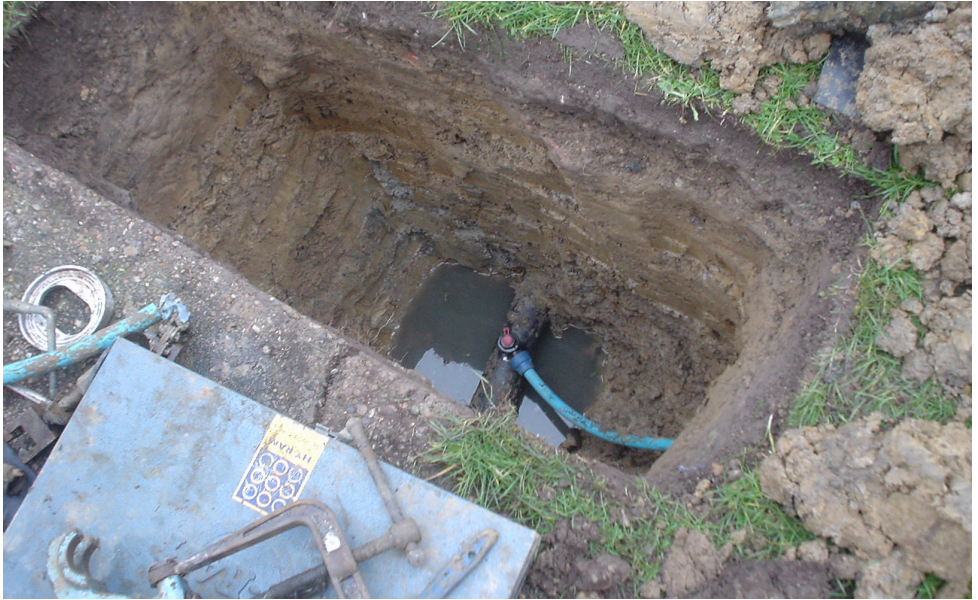
Connection to a main water supply
