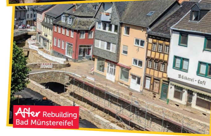
Before Devastation from flooding in Bad Münstereifel
