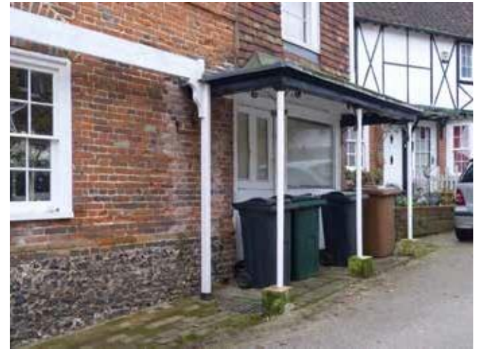
Current bin storage issue
